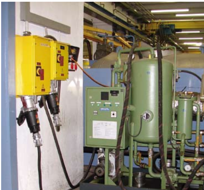
Industry: Oil treatment plant Switzerland
